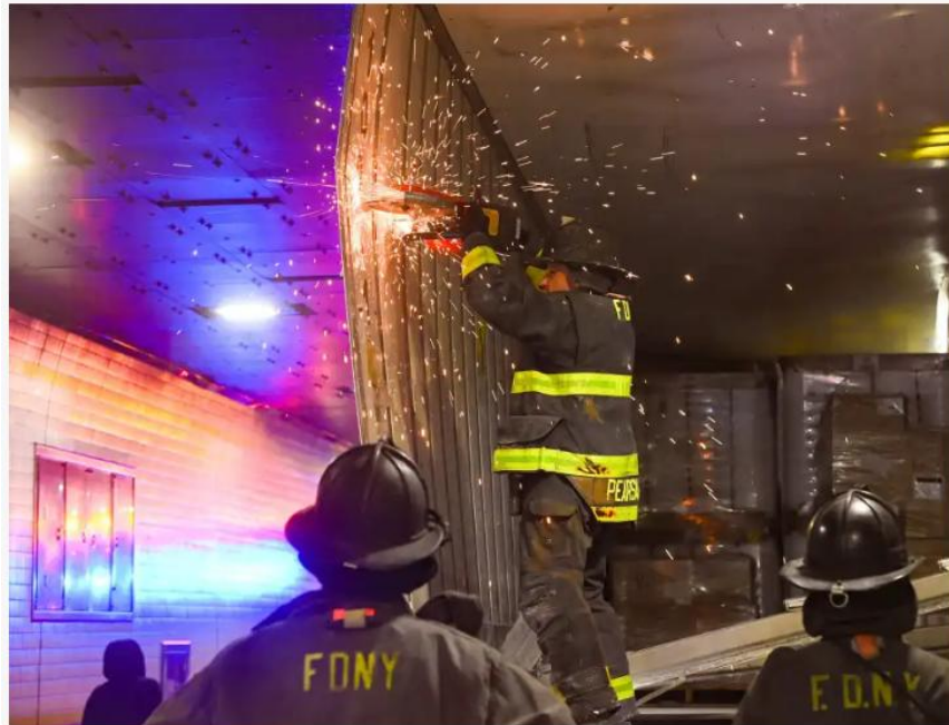
TBTA and FDNY respond to the west tube of the Hugh L. Carey Tunnel where an overheight Manhattan-bound tractor-trailer became stuck on Thursday, Sep 28, 2023. Marc A. Hermann / MTA
